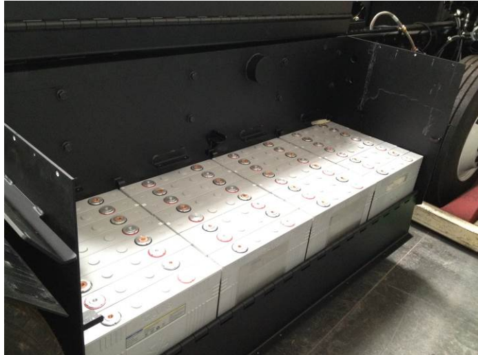
Figure 8. Lower tier tractor battery module housing 32 LiFePO 4 cells.
